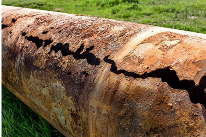
Fig. Pipeline Corrosion, Billion-dollar microbial corrosion issue, S. Simper, World Pipeline, Aug 2022.
